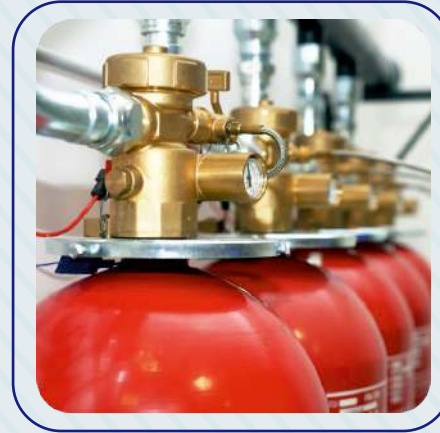
Clean Agent fire Suppression Systems (Fm200,NOVEC,FK5-1-12,C02, InertGas, Aerosole Etc)
